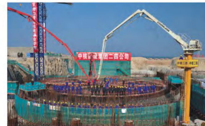
FUQING NUCLEAR POWER PLANT, CHINA 2008 Supply and supervision of PT for containment
